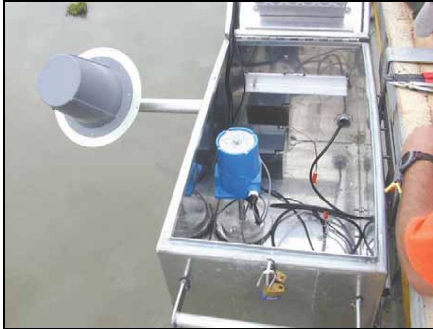
Figure 6. Newly constructed micro-pulse radar, stage-sensor stream-gage at the Notwane River at Mochudi, Botswana.
