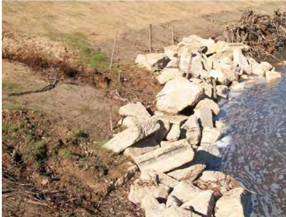
Figure 7. Rock at toe of slope.
