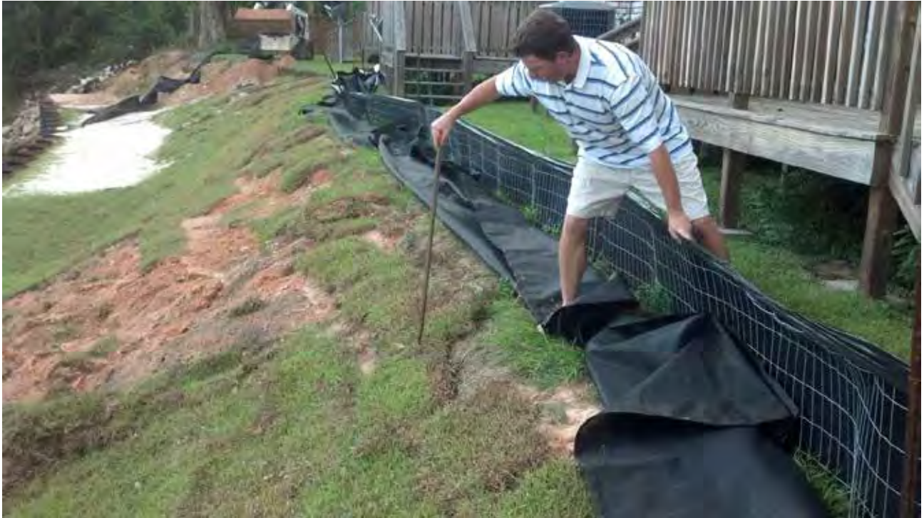
Figure 11. Flooding from the Tchoutacabouffa River caused substantial scouring to the cut bank behind the Riv-erbend Cove Apartments just off Lamey Bridge Rd. A resident (pictured), who stayed during most of the flood event, indicated the high water level to the NWS flood survey team which they used to help estimate the crest for Tchoutacabouffa River at Lamey Bridge Rd (DIBM6).
