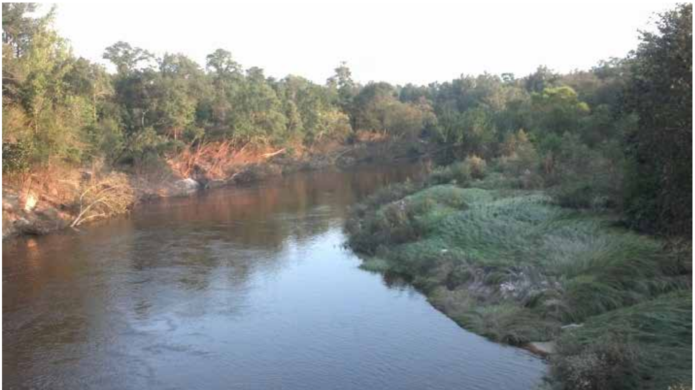
Figure 6. Downstream view from Cable Bridge Rd. Widespread damage to trees and brush were noted.
