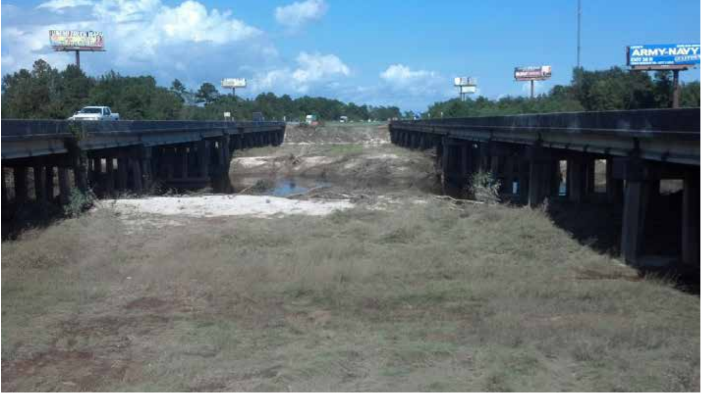
Figure 7. Wolf River floodplain between the eastbound and westbound bridges of I-10. Widespread tree/brush damage was noted along with scouring of the overbank areas.
