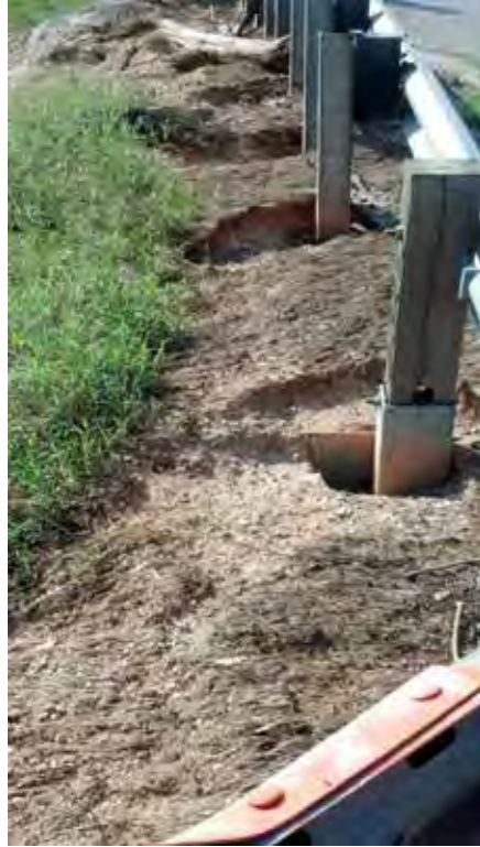
Figure 5. Guardrails on downstream side of the Silver Run Rd. bridge showing evidence of scouring.
