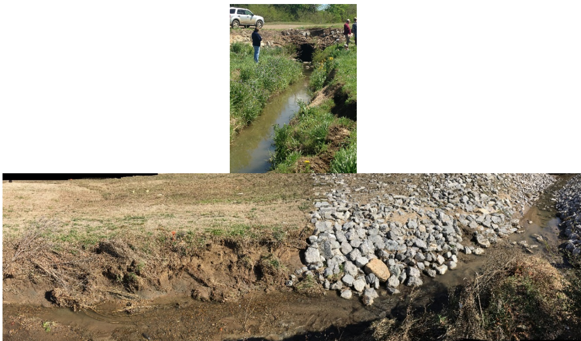
Figure 20. Progressive streambank instabilities and erosion after removal of culvert at the joint of a headwater tributary with main stream of Catalpa Creek.
