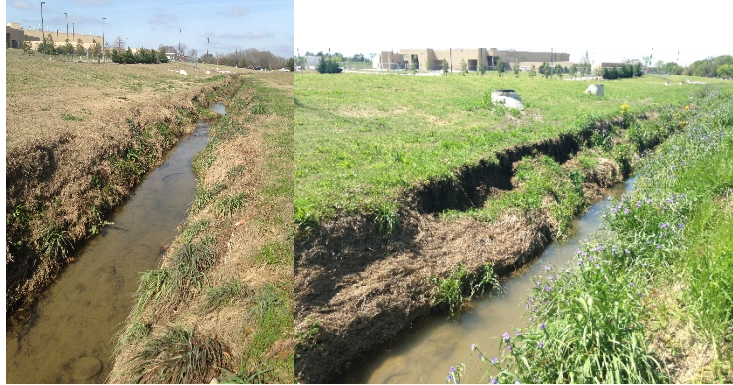
Figure 21. Planar failure along headwater tributary
