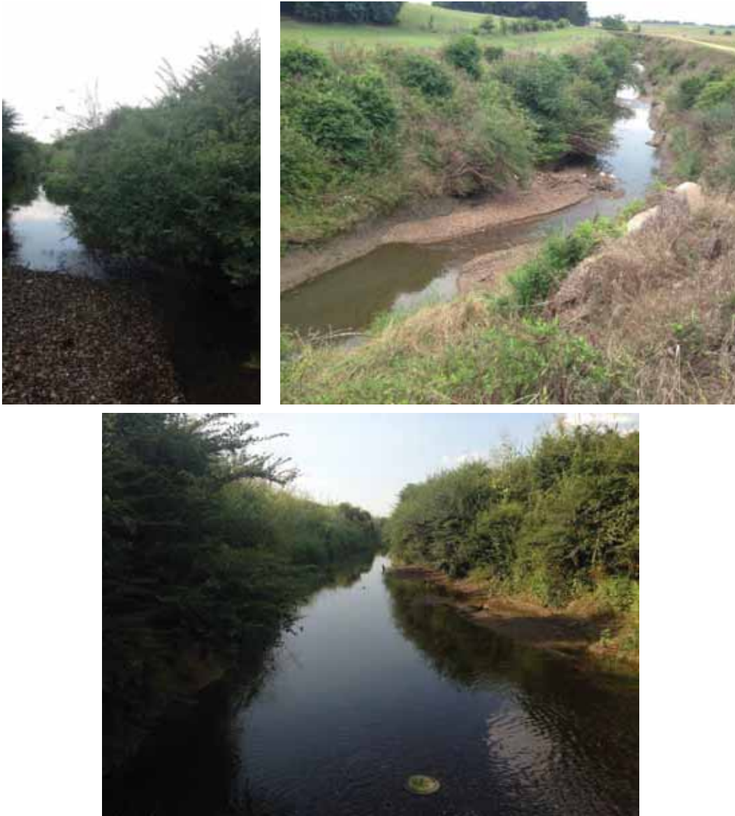
Figure 9.1.8. Sand and gravel bars formation along internal sides of bendways, upstream of streams junction and stream segments with abundant vegetation along the main stream of the Red Bud – Catalpa Creek Watershed.
