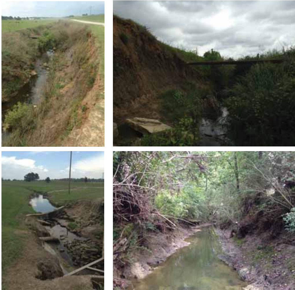
Figure 9.1.7. Evidences of low sinuosity, active unstable streambanks, undercutting and streambed erosion/outcrop along the main stream and below a hydraulic structure in a tributary of the Red Bud – Catalpa Creek Watershed.
