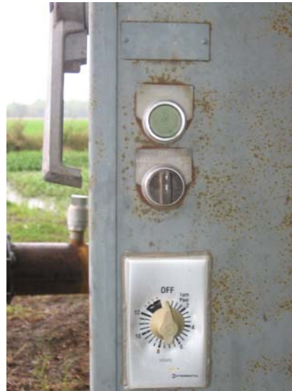
Figure 7. Manual timers installed to control irrigation pumps can save additional water and energy in soybean and rice production.
