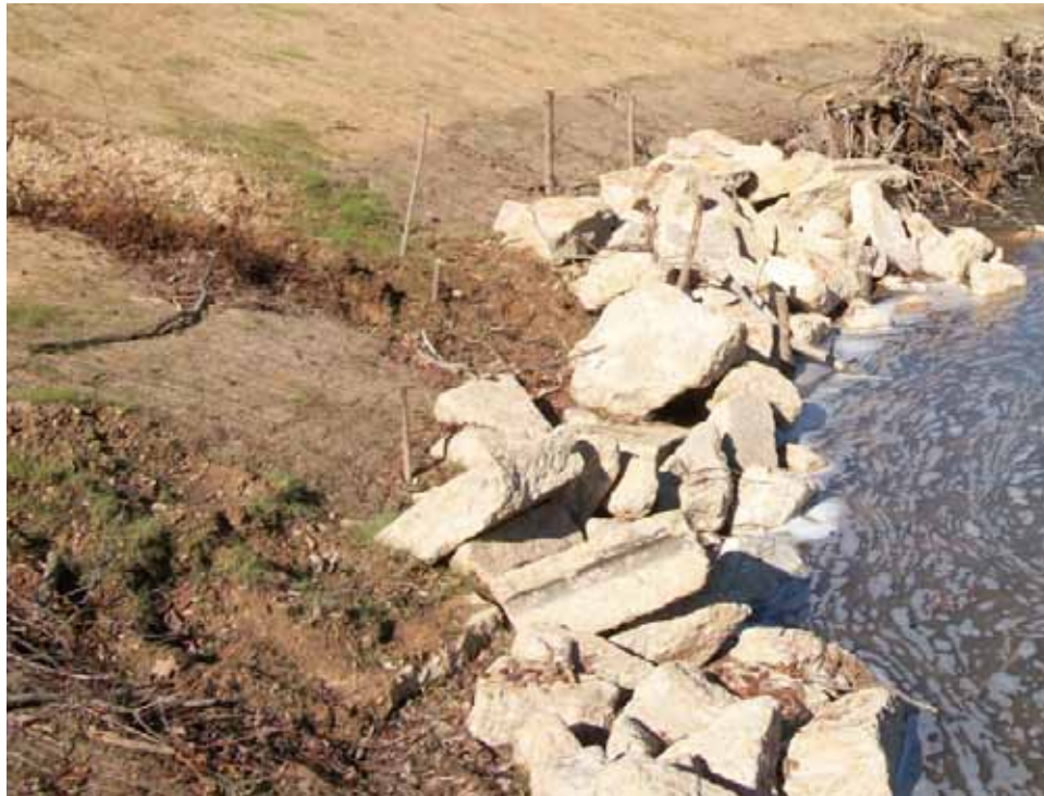
Figure 7. Rock at toe of slope.
